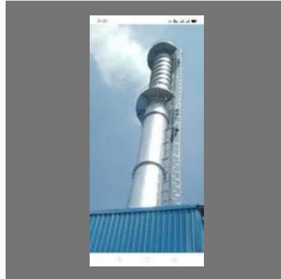
10 Mm Mild Steel Chimney
