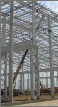
MS Prefabricated Structure Service
