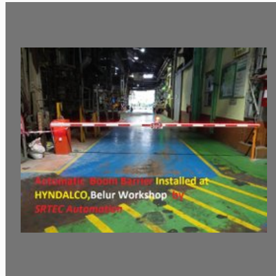
Parking Access Control Systems
