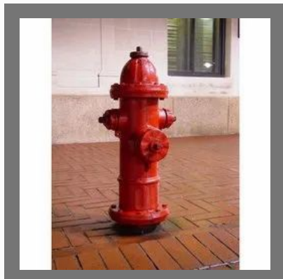
Outdoor Fire Hydrant
