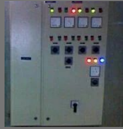
Electrical Works With Supply
