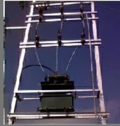
Residential Electrical Works
