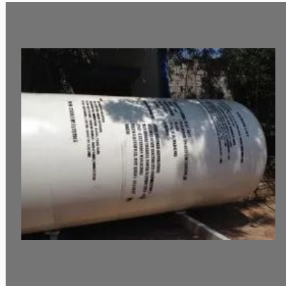
Chemical Storage Tanks
