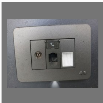
Phone Cable Switch Board
