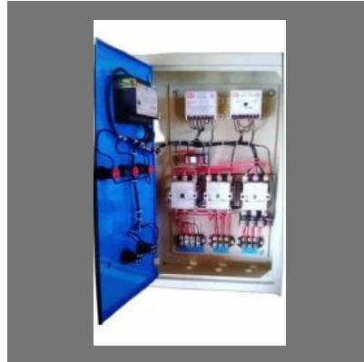
30HP Star Delta Motor Control Panel
