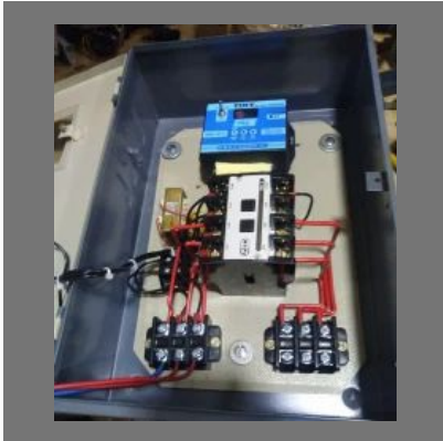
3 Phase Dry Run Control Panel
