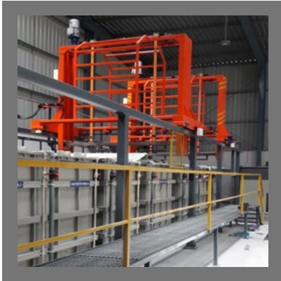
Zinc Nickel Electroplating Plant
