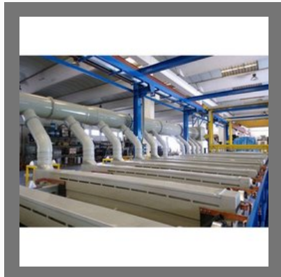
Tin Electroplating Plant
