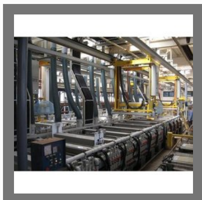
Automatic Zinc Plating Plant
