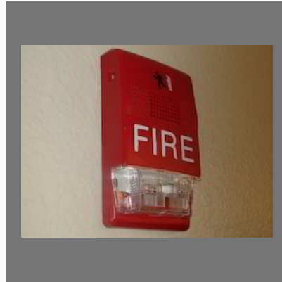
Fire Detection System
