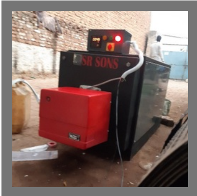
Diesel Fired Boiler 100 kg
