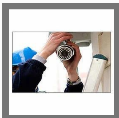
CCTV Installation Services
