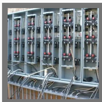
Commercial Electrical Works
