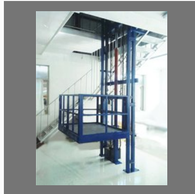
Industrial Goods Elevator
