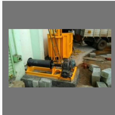
Elevator Gear Box
