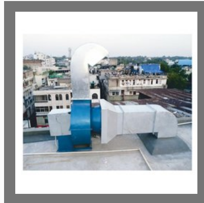
Exhaust Fresh Air Duct
