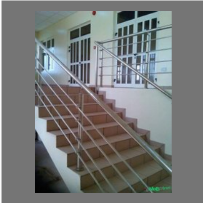
Metal Railing For Stairs
