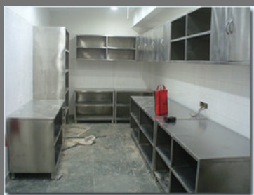
S.s. Work Tables And Overhead Storage
