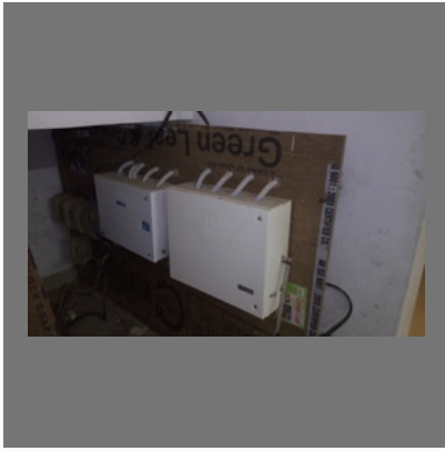
Electric Wiring House
