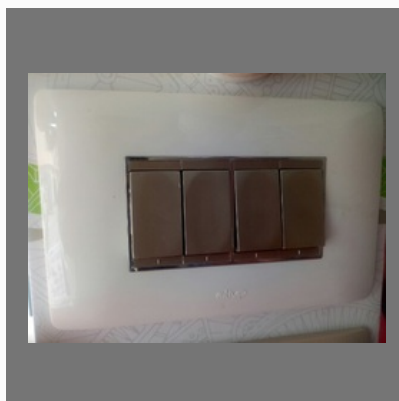
Electrical Switches Service
