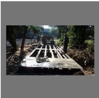
Mild Steel Weighbridge
