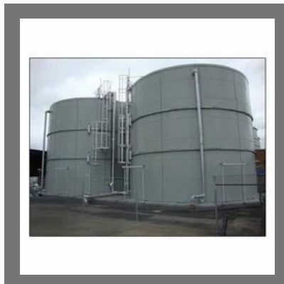
Mild Steel Storage Tanks
