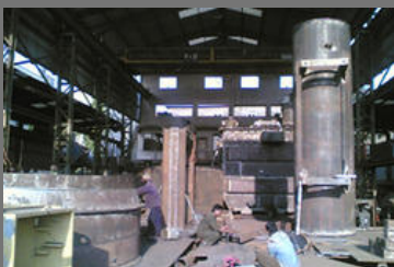
Power Plant Machinery
