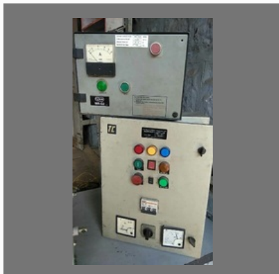
Electrical Engineering Works
