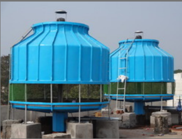
FRP Cooling Tower
