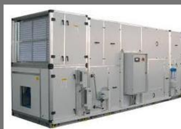
Air Handling Unit & Maintenance Service
