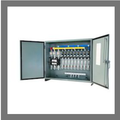
LT Distribution Box with MCCB
