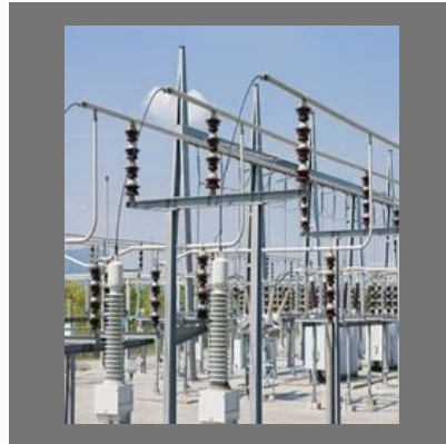
Industrial Electrical Contractor Service
