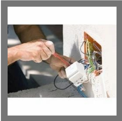
Home Electrical Maintenance
