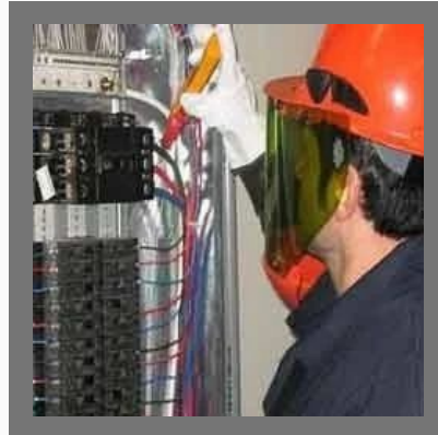
Hotel Electrical Maintenance
