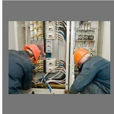
Commercial Electrical Contractor Service
