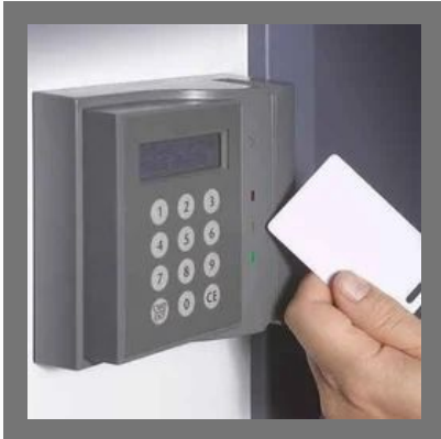
Proximity Access Control System
