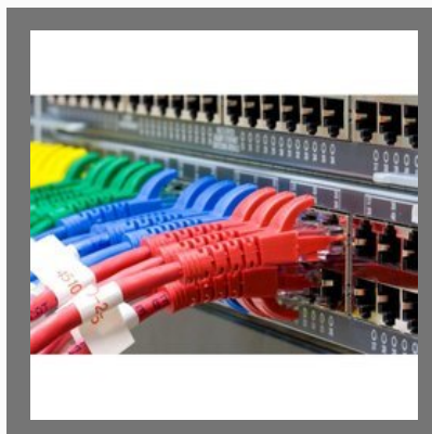
Voice Cabling Service
