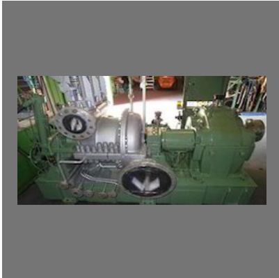
Process Steam Boiler EPC Service
