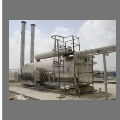
Indirect Water Bath Heater
