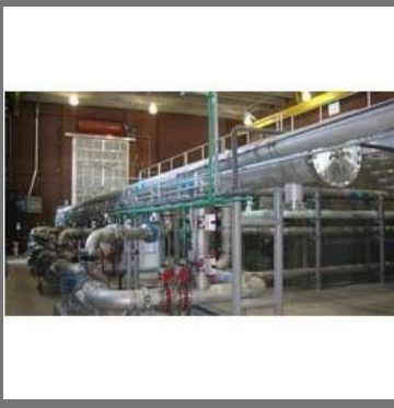
Membrane Water Treatment Plant
