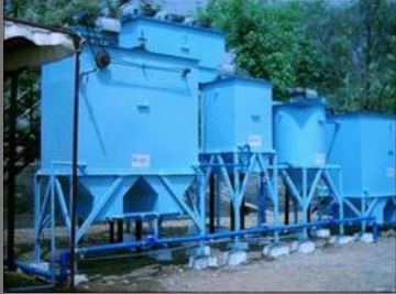
Effluent Treatment Plant
