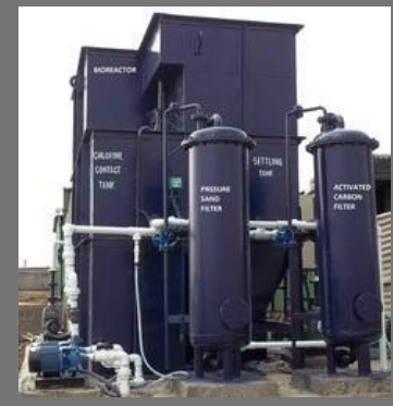
Sewage Recycling Plant
