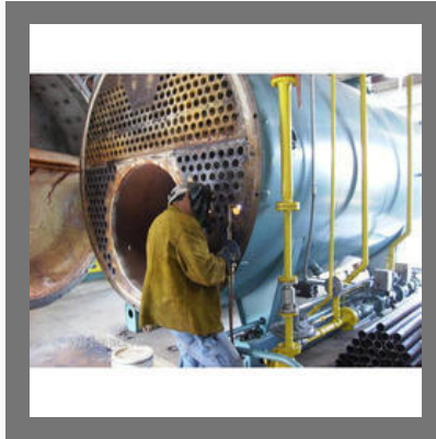
Steam Boiler Installation Service
