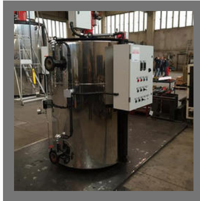
Diesel Fire Thermo Pack Boiler
