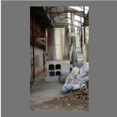
Thermic Fluid Boiler
