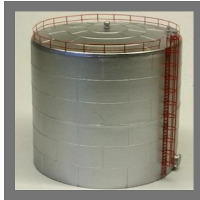
Oil Storage Tank
