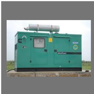
24 hours power back up
