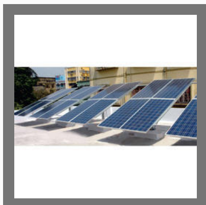
Solar On- Grid System
