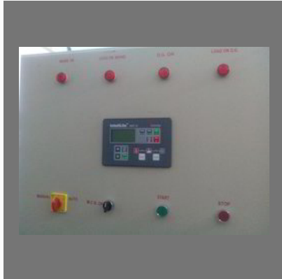
Electrical AMF Panel
