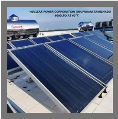
INDUSTRIAL SOLAR WATER HEATERS
