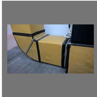
Air Channel Ducting
