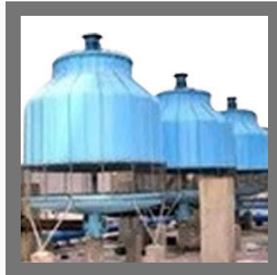
Cooling Towers Heat Exchangers
