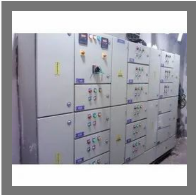
LT Electrical Panel Installation Service
