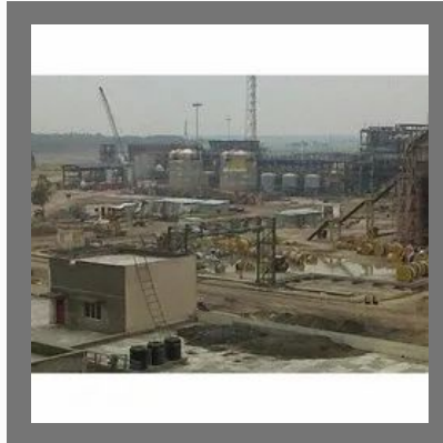
Electrical Installation Service
