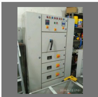
Electrical Industrial Panel
