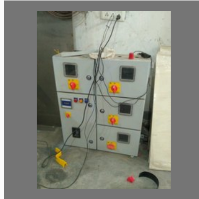
Electric Control Panel
