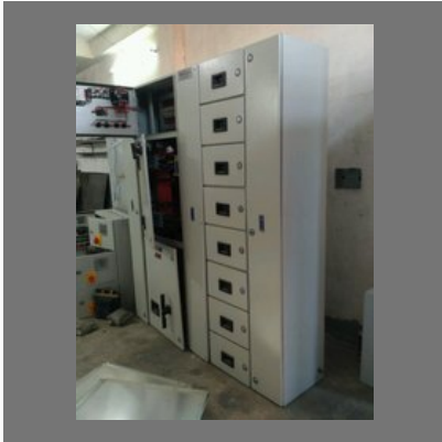
Corporate Electrical Panels
