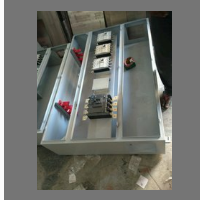
Electric Control Panel
