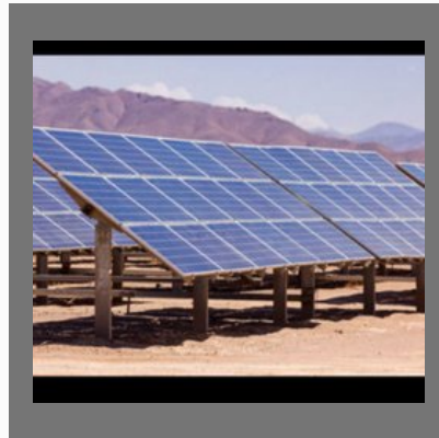
On Grid Solar Power System
