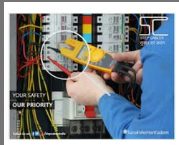
Hospital Building Electricals Services
