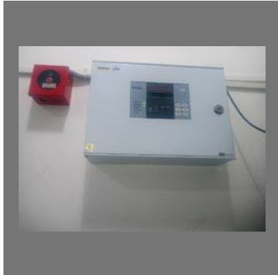
Fire Alarm Signaling Device
