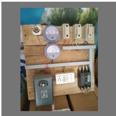
Switch Board For Agricultural Pump
