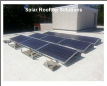
Solar Rooftop Solutions
