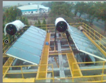
Solar Water Heating System
