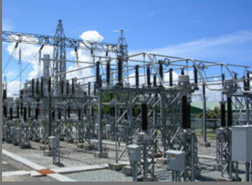
Sub Stations Maintenance
