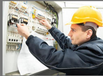
Electrical AMC Services
