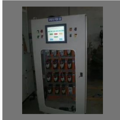
Automation Control Panel
