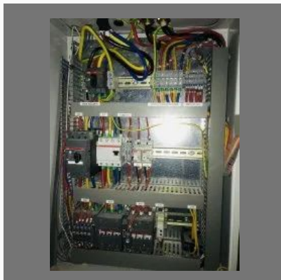
Ahu Control Panel
