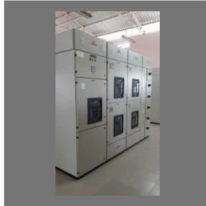
Power Control Centre
