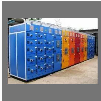
PCC Panel Board
