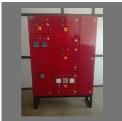
VFD for Fire Fighting Panel
