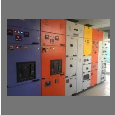
Lt Switchgear Panel
