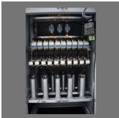
APFC Panel - AUTOMATIC POWER FACTOR PANEL
