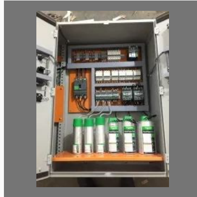
Automatic Power Factor Capacitor Panel
