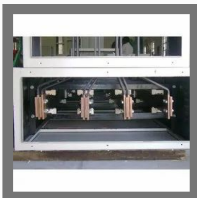
LV Bus Duct
