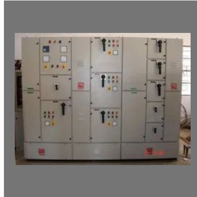
Lt Distribution Panel
