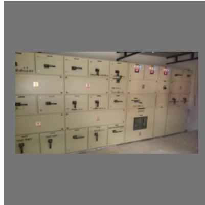
Power Distributions Panel
