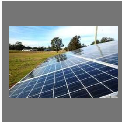
Off Grid Solar Power Plant
