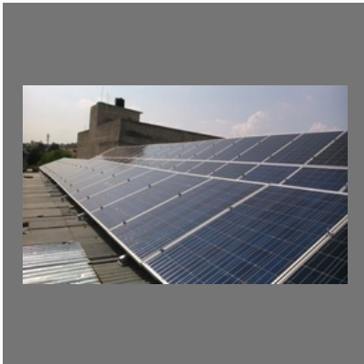
On Grid Solar Power Plant
