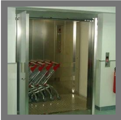
Mall Freight Elevator
