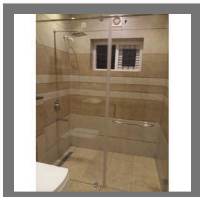
Glass Shower Cubicles
