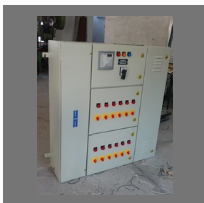
Automatic Power Factor Panel
