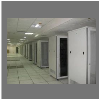
Raised Flooring Anti Static Laminate Finish
