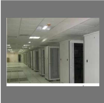
Anti-Static Server Room Raised Flooring
