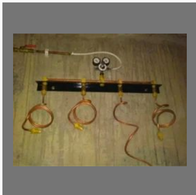
Oxygen Manifold System
