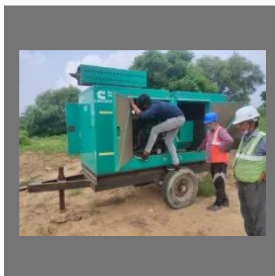
Diesel Generator Annual Maintenance Service
