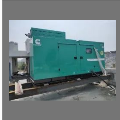
Silent Diesel Generator Service
