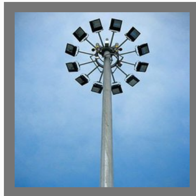
High Mast Lighting
